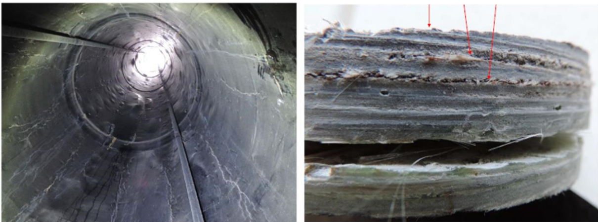
Figure L9. Severe delaminations seen as large buckles in a flue gas stack. L10. Cross-section of a delaminating FRP from a flue gas stack.
