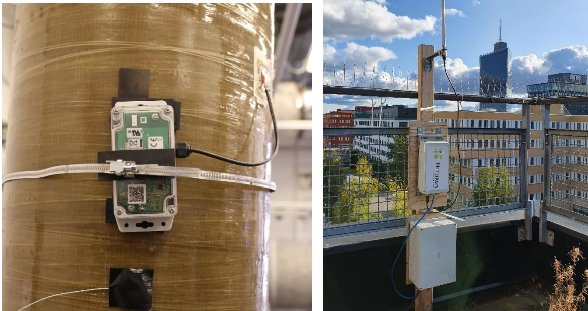
Figure L2: The sensor housing containing the radio sensor with a connected piezo crystal mounted on an FRP-construction. Figure L3: The gateway installed on the roof of the building communicating with the installed sensors and enable the data online.
