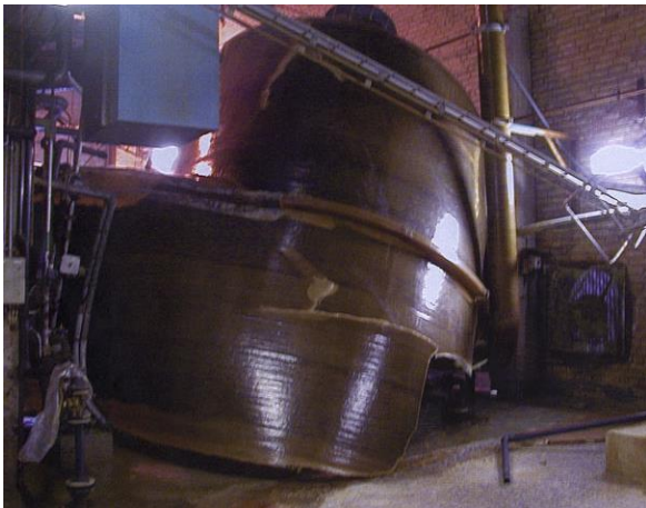
Figure 1 Catastrophic failure of a 60 m 3 spent acid tank made of glass-fibre reinforced polyester (FRP) with a CPVC lining.
