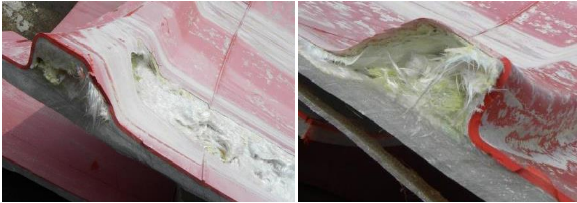
Figure 30. A PVC lined FRP tank for hypochlorite at a chlorine plant. The pH is normally kept high (above 10) but had varied locally which resulted in radical attack from HClO and material thinning.
