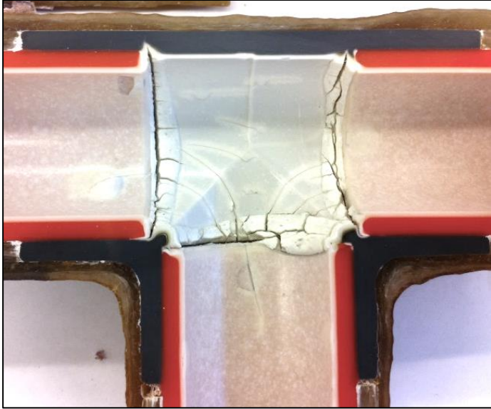
Figure 27, a failed socket cemented weld in a PVC line used for spent acid
