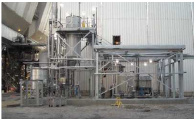
Figure 7.2. PDP process installation at RockTenn mill in Demopolis, USA (Mathis and Futterer 2013)
